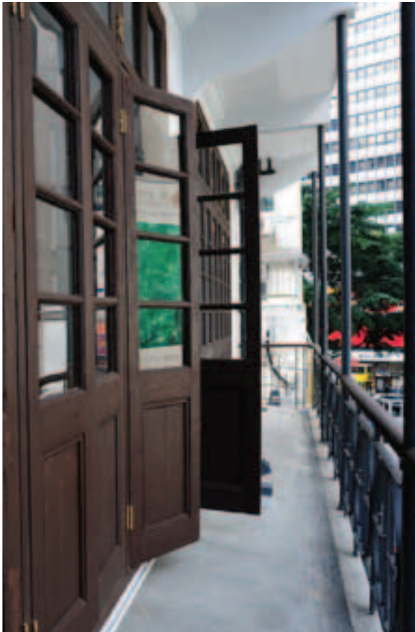
■ The project retains and preserves the character defining elements in pre-war historical buildings.
