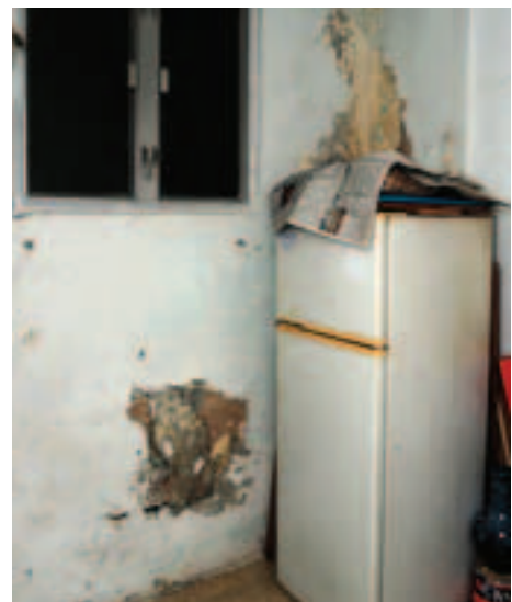
■ Poor building condition at the project site.
