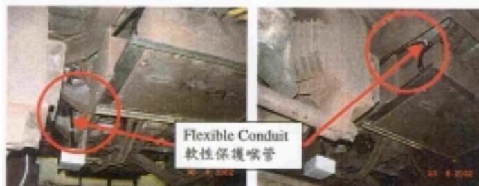
Photo 4 - Flexible Conduit and TDI Trip Switch Junction Box (After Modification) 相片四 - 軟性保護喉管和車鉤脫卡跳脫閘閘製連接盒(修改後)
