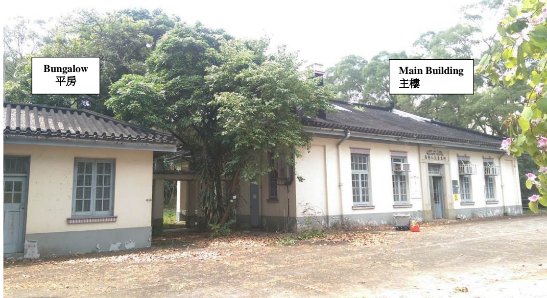
Existing Condition of the Lady Ho Tung Welfare Centre 何東夫人醫局主樓及平房的現貌
