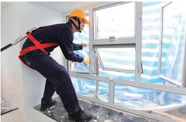
「職安健星級企業—裝修及維修業安全認可計劃」已推廣至供50人或以上的非中小型企業申請。 “OSH Star Enterprise – RMAA Safety Accreditation Scheme” expanded its services to Non-SMEs with 50 employees or more.
