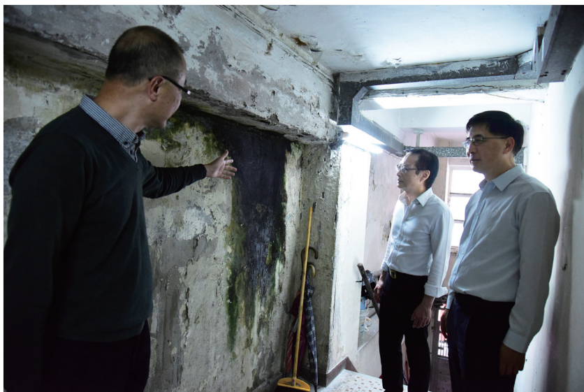
Visiting the Oak Street/Ivy Street project on the day of project launch and inspecting the varied and poor building condition with URA staff members.
