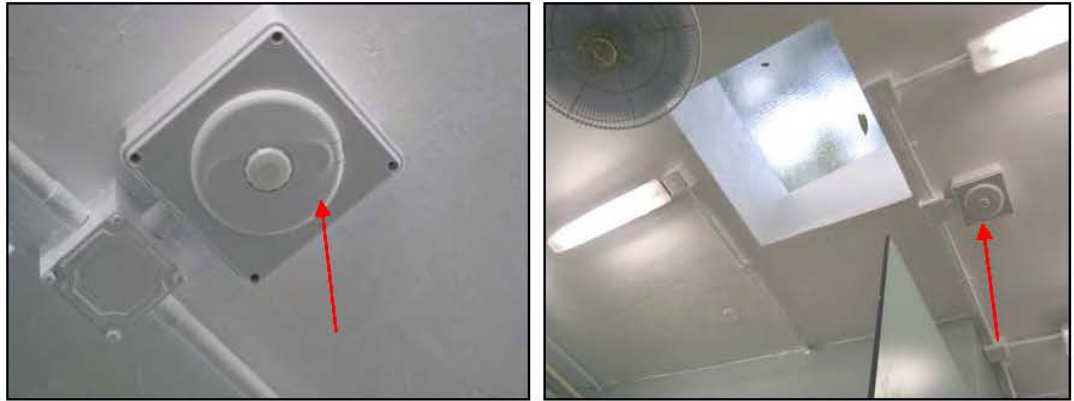
Motion sensor control installed inside toilet
