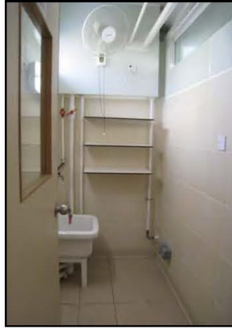
Slop sink and storage facilities inside a compartment
