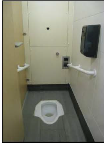
Cistern and related piping are concealed from view, leaving the toilet cubicle clean and tidy
