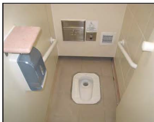
Squatting type water closet
