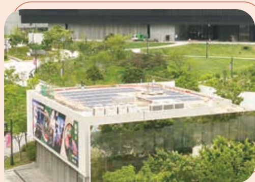
The new photovoltaic system installed on the roof of Freespace 自由空間天台新設的太陽能光伏系統
