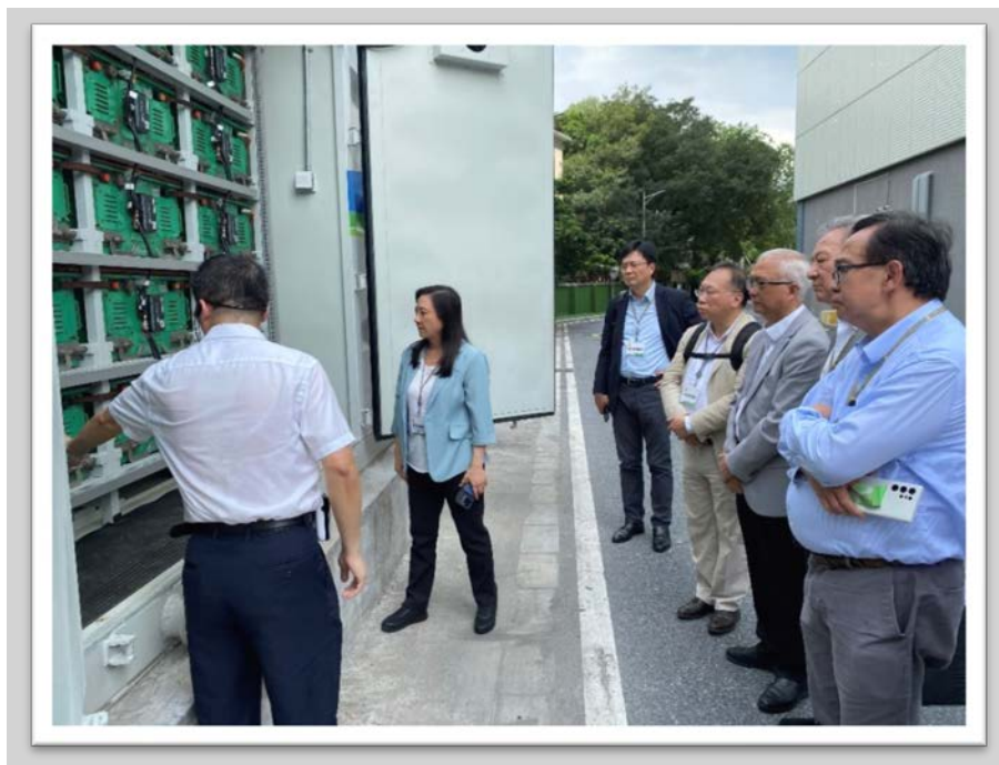
Staff of the Yangling new energy eco-industrial park briefs the Delegation on the outdoor cascade battery energy storage facilities
