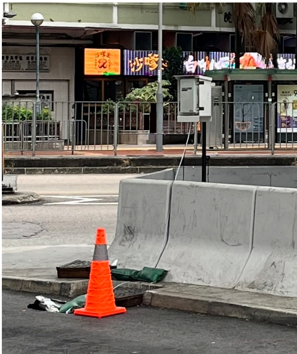
Trial installation of odour monitoring equipment at stormwater manholes to support the surveillance cameras system.
