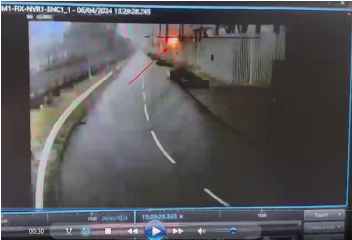
Figure 3 Discharge of around 0.6 seconds at C5 Generator Transformer Compound
