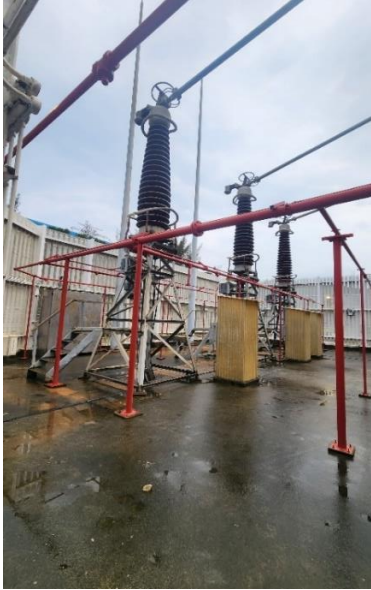
Figure 6 C5 Generator Transformer Compound after Voltage Dip on 6 April
