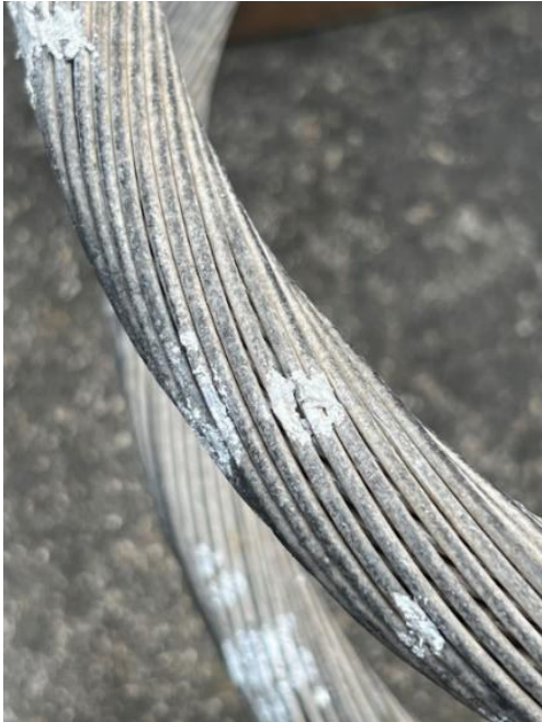
Figure 13 Localized Burn Marks at Flexible Conductors of C6
