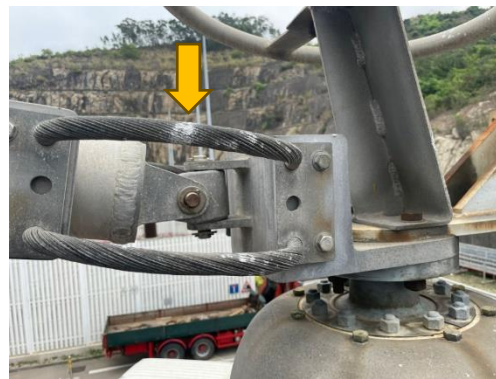
Figure 16 C6 Damage at Flexible Conductor near HV Outlet
