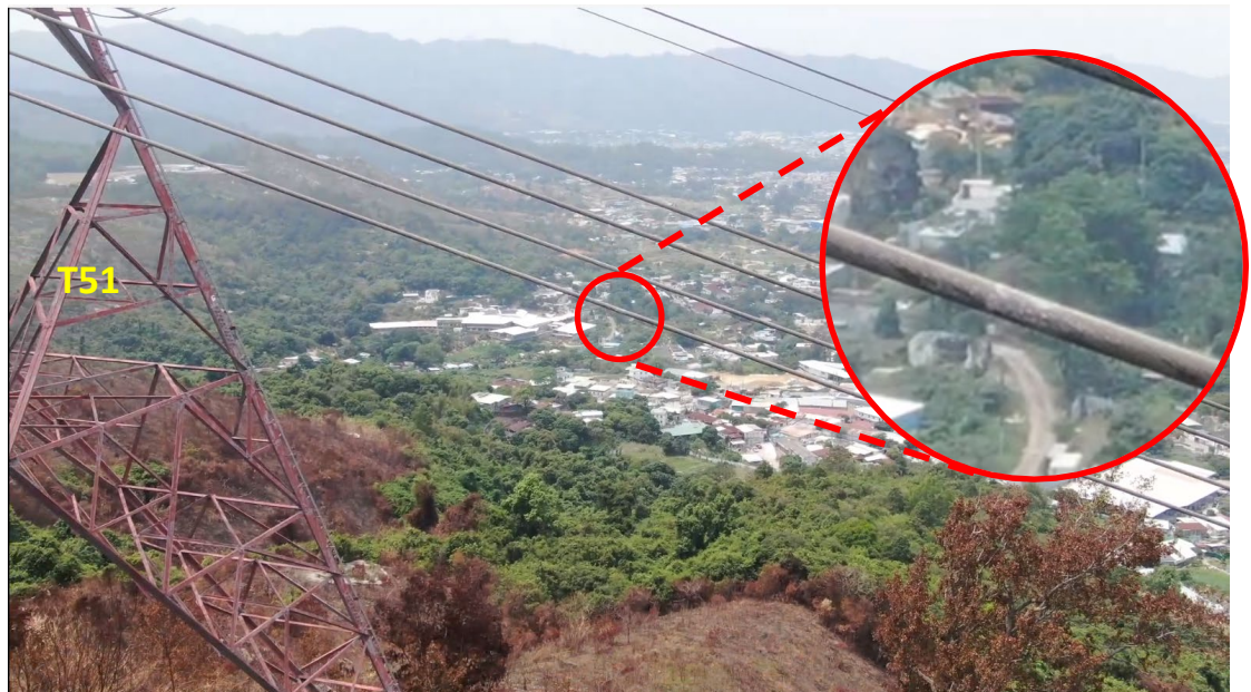
Figure 2: Flashover marks on L3 phase conductor near T51
