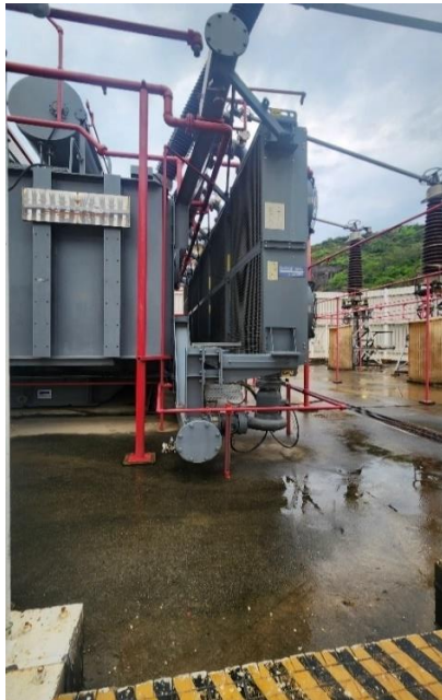
Figure 8 C6 Generator Transformer Compound after Voltage Dip on 6 April
