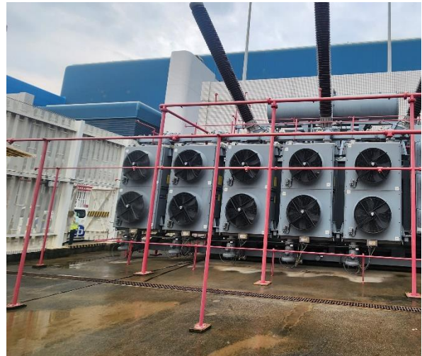
Figure 9 C6 Generator Transformer Compound after Voltage Dip on 6 April
