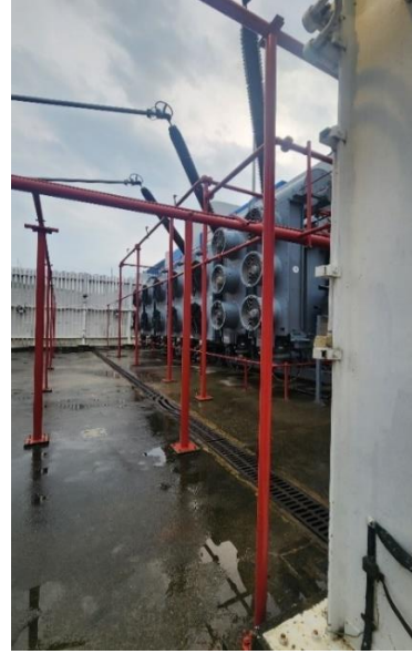
Figure 7 C5 Generator Transformer Compound after Voltage Dip on 6 April
