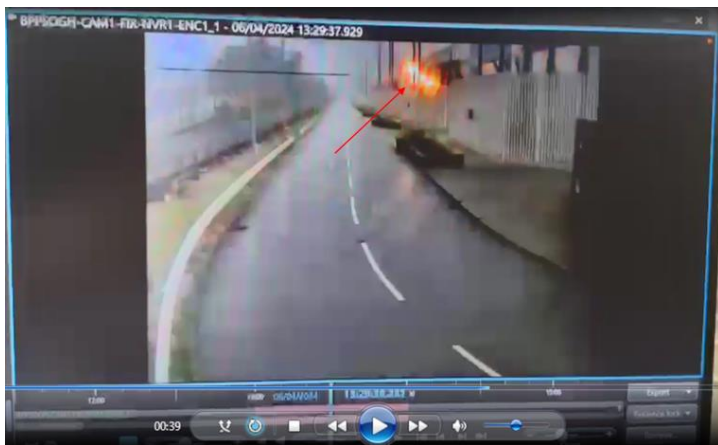
Figure 5 Discharge of around 0.8 seconds at C6 Generator Transformer Compound
