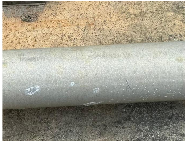
Figure 12 Patches of Metal on C5 HV Jumper
