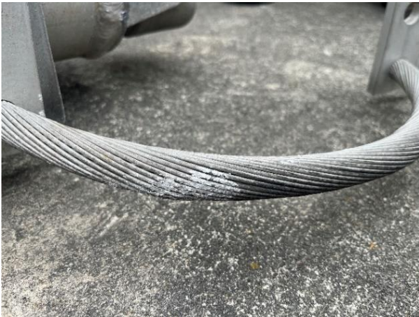
Figure 11 Localized Burn Marks at Flexible Conductors of C5
