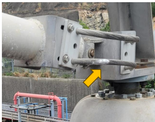
Figure 15 C5 Damage at Flexible Conductor near HV Outlet
